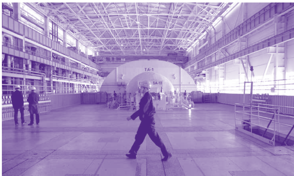
Inside the turbine hall at unit 1 of the Zaporizhia nuclear plant, one of 12 Soviet-era nuclear units up for lifetime extension in Ukraine.
